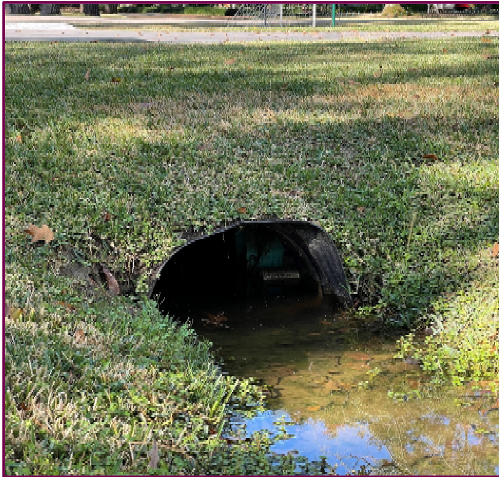
Figure 4. Obstructed pipe underneath driveway culvert with two drainage pipes cutting into it.
