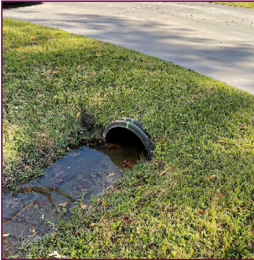
Figure 2. Recent Ponding in Ditch.
